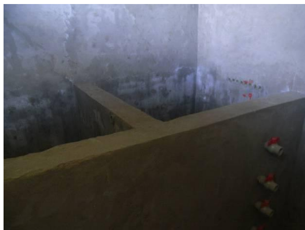
The runoff holding tank
